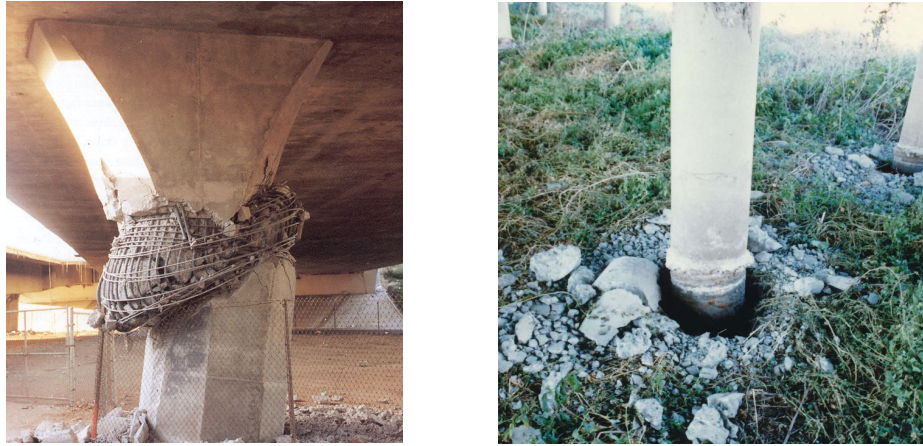
Figure 3. (a) Shear failure of a column with a flare in Northridge earthquake (Mitchell et al. [11]) and (b) column in pile bent embedded in soft soil showing soil-structure interaction (Mitchell et al. [12]).
